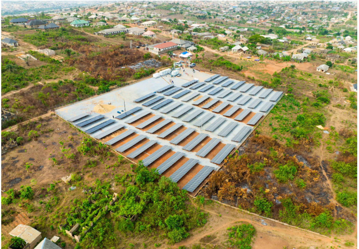
Robinyan IMG generation plant.
