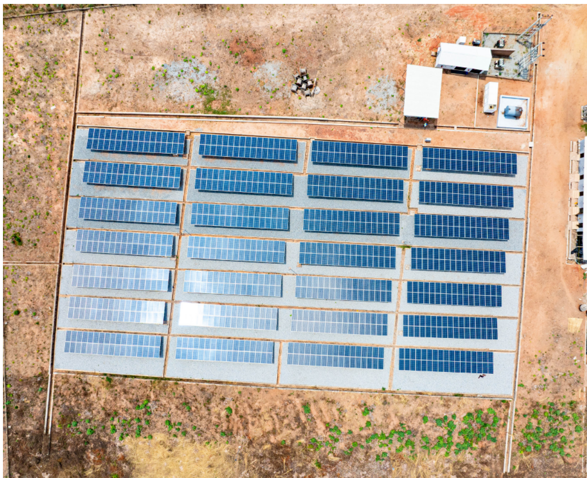
Toto IMG generation plant.
