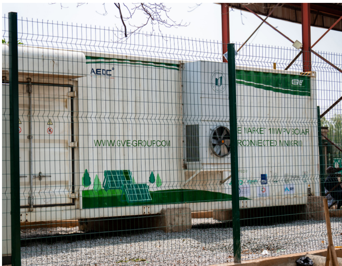
BESS in Wuse IMG.
