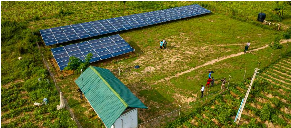
Drone footage of a minigrid in Gwam, Niger state. Photo credit: TNF Media
